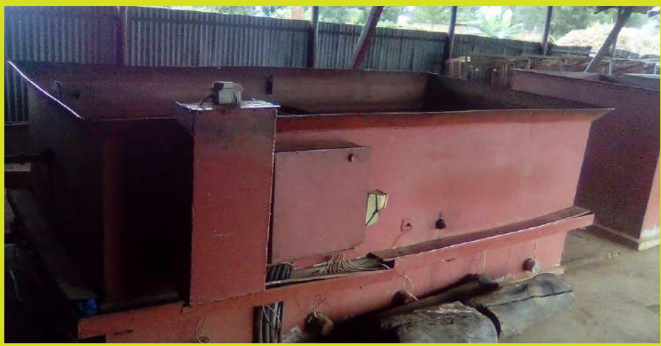
Hot water treatment trays
