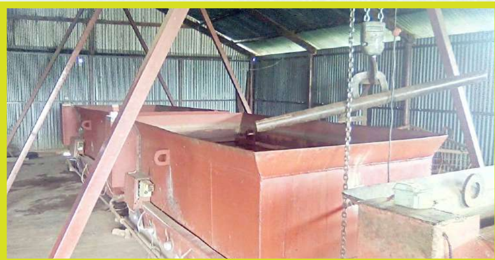
Hot water treatment plant
