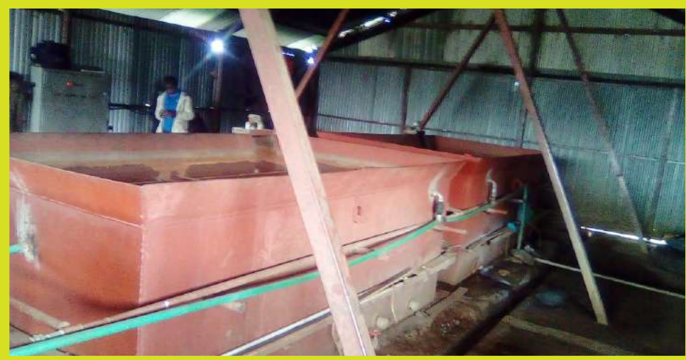
Hot water treatment plant
